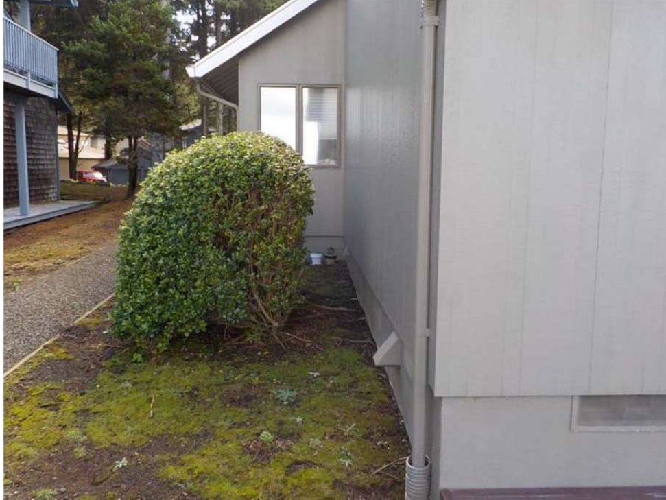
Photo 3 – View along the northeasterly side of the house, in the area of proposed construction.
